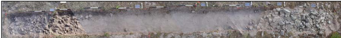
Figure 19. View showing rubble from collapsed gabions/fascines at east and west ends of trench.
