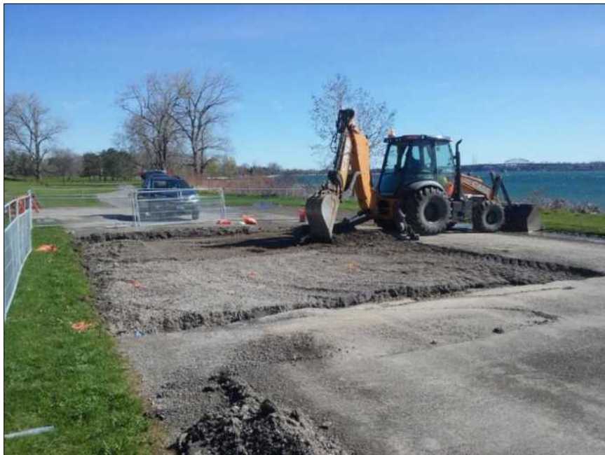
Figure 192. View looking northeast showing the upper 10-15 cm of gravel bedding below the asphalt being removed by machine.
