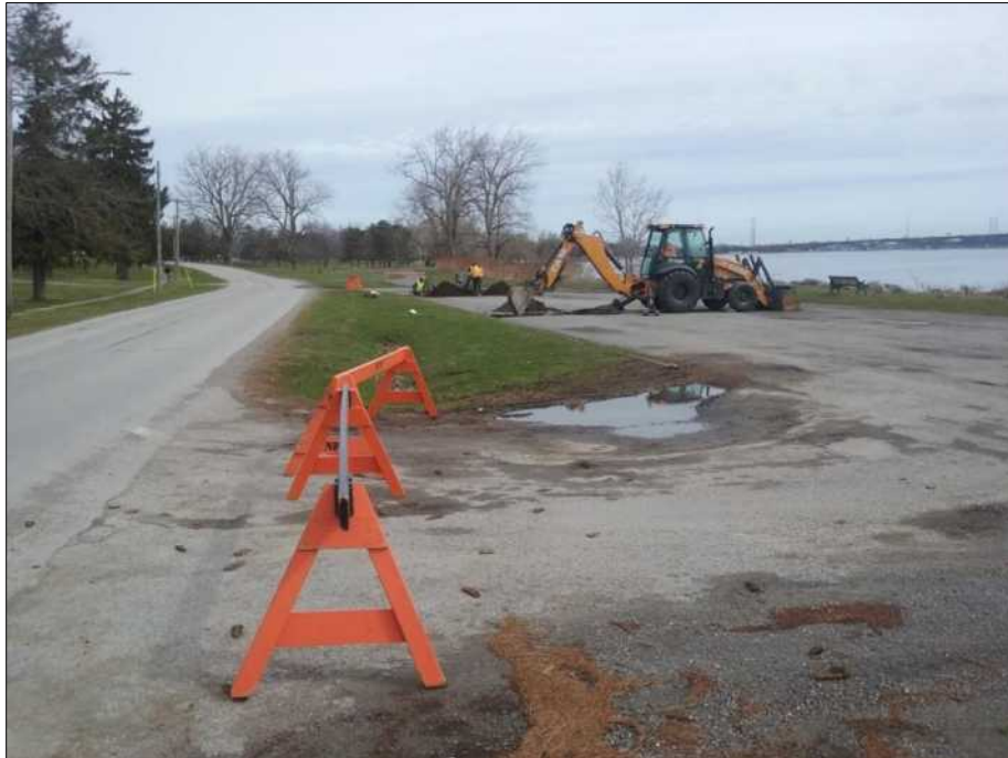
Figure 18. View looking north showing parking lot between Lakeshore Road and the Lake Erie shoreline. Excavation in progress for Trench 2. Trench 1 complete.
