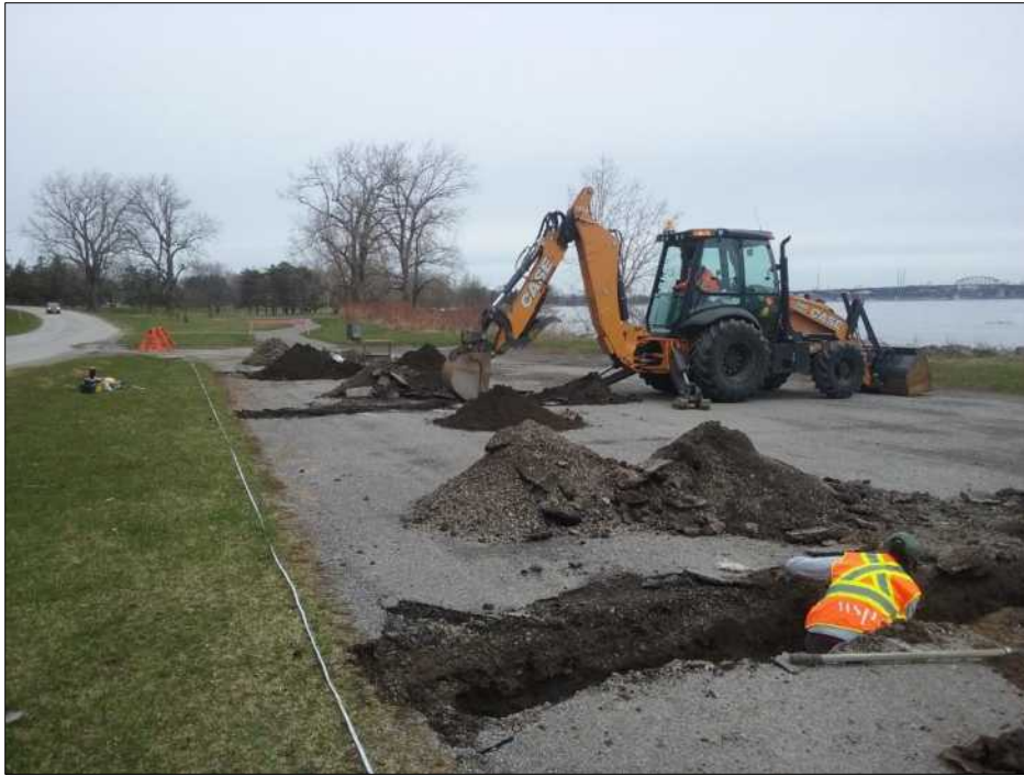
Figure 19. View looking north showing three trenches excavated on April 16 to verify GPR survey results of October 30, 2018. Trench 2 is in foreground and Trench 1 in background. Trench 3, in the middle ground, is under excavation.
