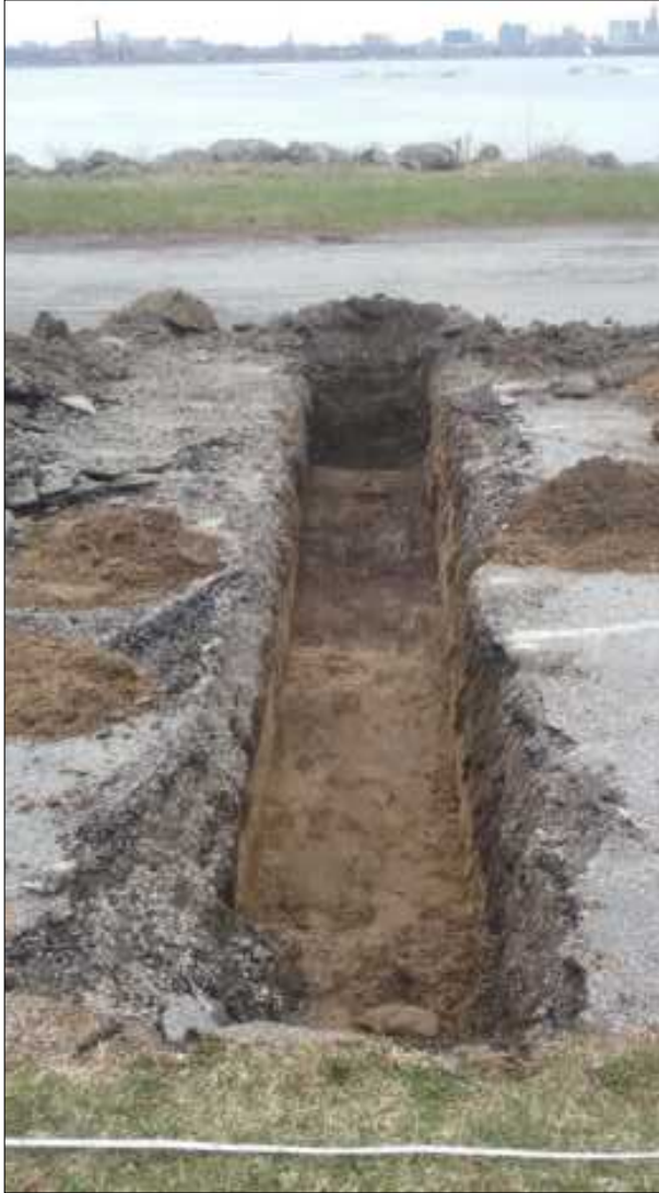
Figure 31. Trench 3 view looking east showing dark stain in subsoil in east end of trench.
