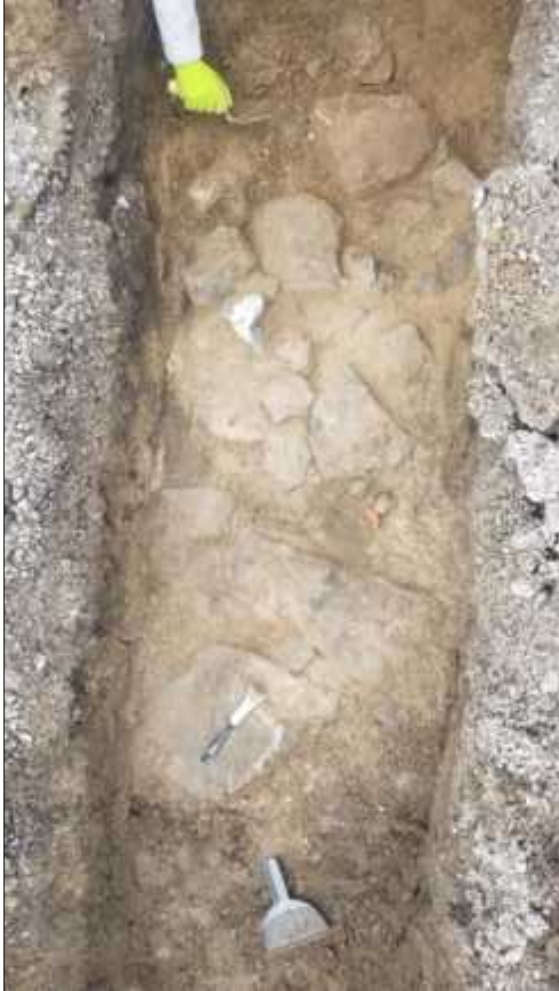
Figure 29. Trench 2 overhead shot of wall foundation and collapse being exposed by hand excavation.
