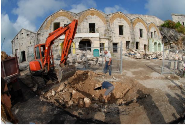
Figure 2 Machine excavation of the Lower Ordnance yard to remove the deep fill between the 'North Building' and the tunnel entrance. 'Johnny' Bernard supervising, Andrew Harris excavating.
