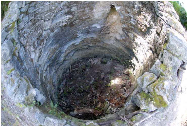
Figure 5 View inside kiln showing debris and collapse that has accumulated on the kiln floor to a depth of between 1 and 2 m.
